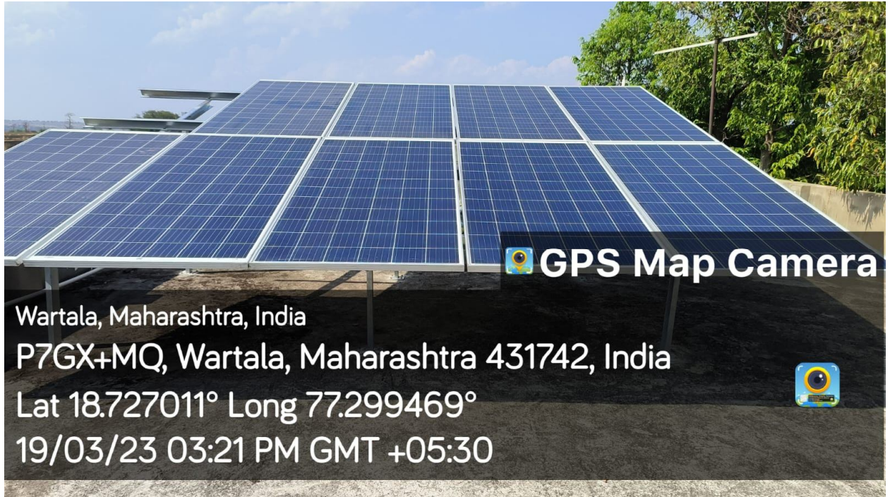
Ongrid Roof Top Solar System (3KW) on Roof
